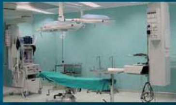
Emergency Lighting & Energy Stations
